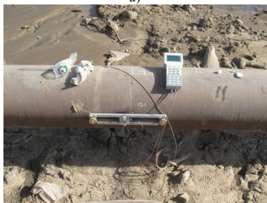
Fig. 2. Installation diagram for the primary instrument, a , and the general view of the flow meter installed on the inlet line, b .
