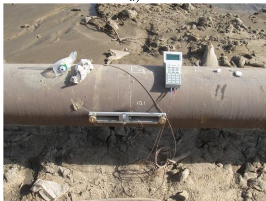
Fig. 2. Installation diagram for the primary instrument, a , and the general view of the flow meter installed on the inlet line, b .
